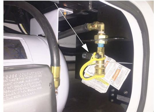
LP Accessory Connection (Located inside propane tank compartment on passenger side of motorhome) -Typical View
