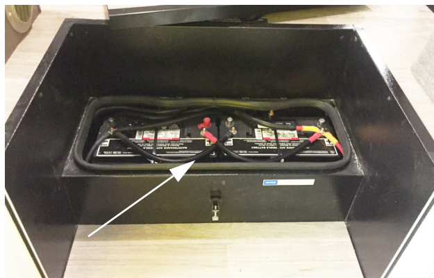
House Batteries (Entrance Step Removed) -Typical View
