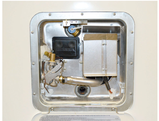
Water Heater Exterior Service Access
